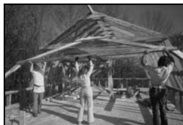
David Maynard, Terry, and Roger Crockett putting up rafters on the first part of the shop building in 1980
